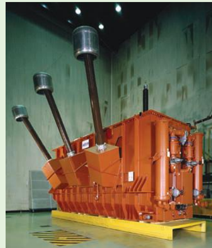
Figure 44.5 Step-up transformers at a power station
