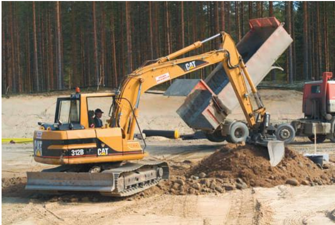
Figure 16.7 A hydraulic machine in action
