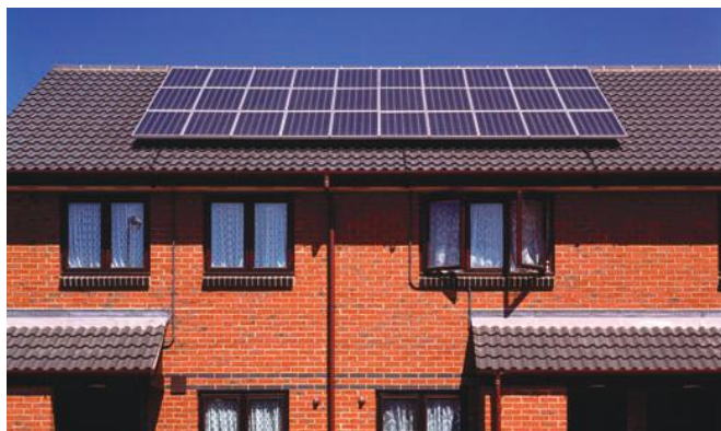
Figure 15.1 Solar cells on a house provide electricity.
